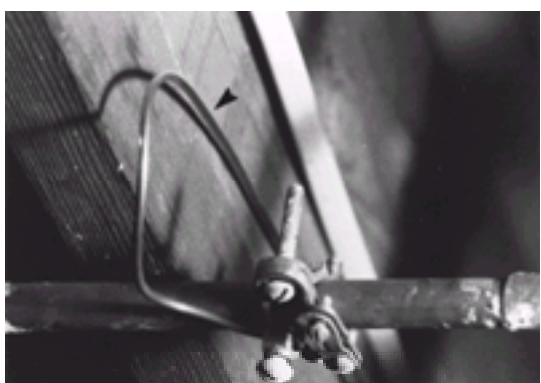
Figure 8-8. The arrowhead indicates the ground wire from the fuse box attached to a cold-water pipe.
