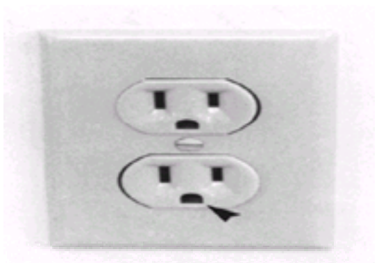
Figure 8-11. Modern electrical outlet in which the ground wire is present. The arrowhead points to the part of the receptacle where the ground wire connects.
